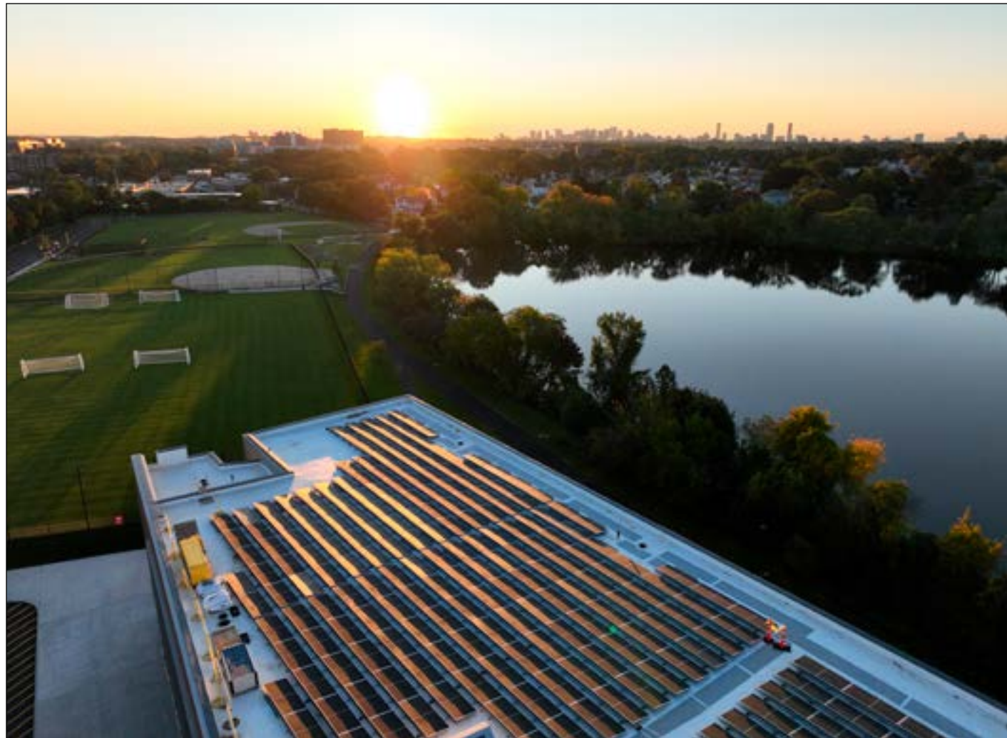
Rooftop solar array at Belmont Middle and High School.
